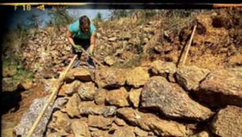
Schools were organized to learn the technique of dry-stone wall construction, targeting local people
